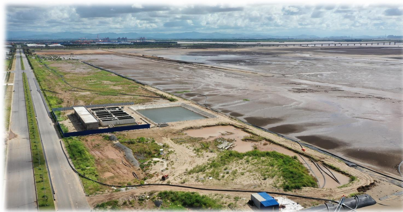
The new technical hub area is gradually taking shape, and an additional 280 hectares of land are being filled and developed for infrastructure
